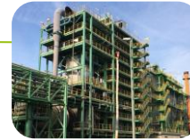
Rotating kiln incinerator
